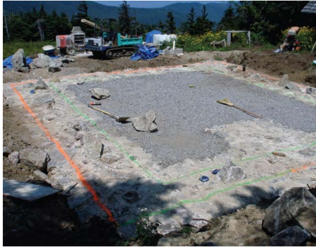
The cabin foundation ready for walls; note protruding stones that will key into the walls.
