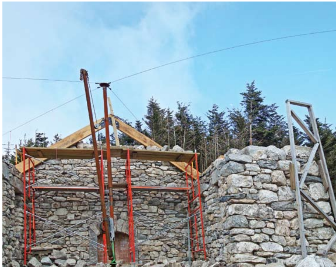
Half a stone cabin. You can see the batter of the walls in the guides we built. The side walls are battered, three feet at the base, two feet at the top.
