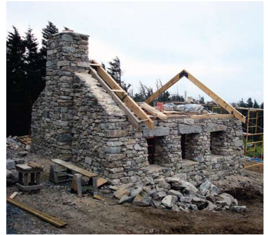
Rear view showing chimney and the first rafters. There are three windows one each side with large granite lintels.
