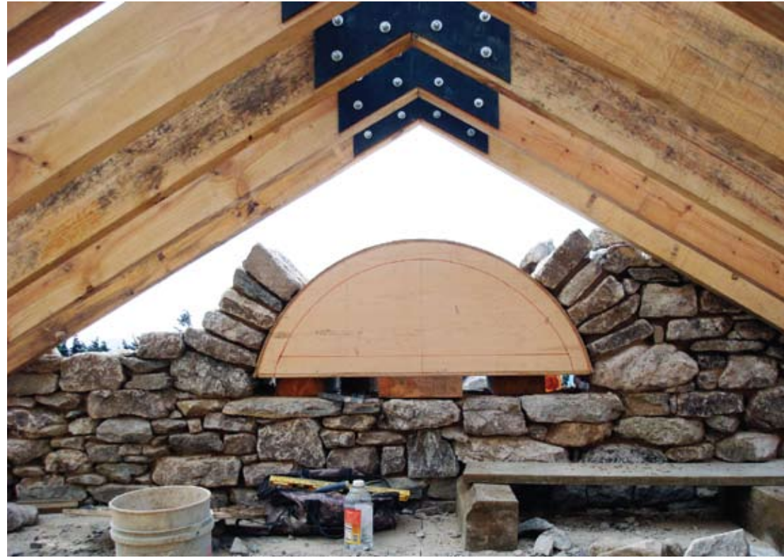
The arch on the cabin face in process. The wall is two feet thick here.
